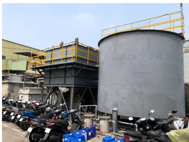
▲ Wastewater treatment facility in the plant
