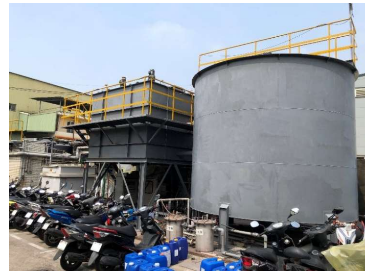
Wastewater treatment facilities
